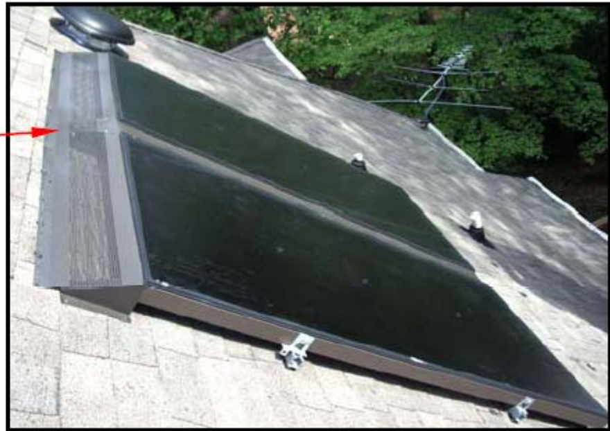
Fig.82 – Two collectors with center-flashing and leaf-guard
