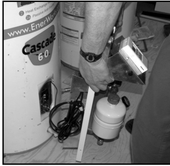
Fig.4.2.6– Positioning Energy Station.
