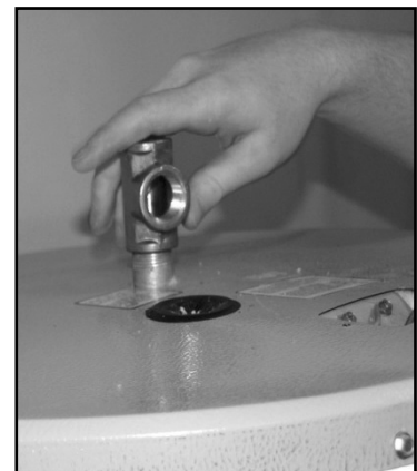
Fig.4.3.1 – Brass tee connected to top of solar storage tank
