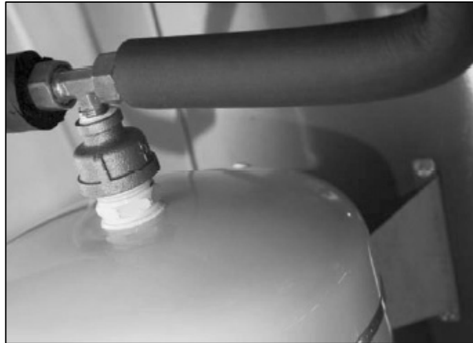
Fig. 4.9.2.2 – Supplemental expansion tank in line from top of heat exchanger to collector.
