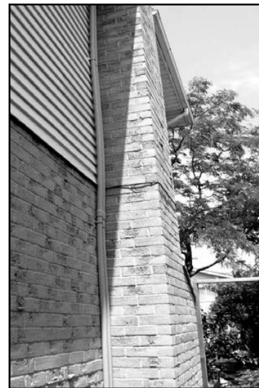
Fig. 4.2.3 – Exterior line-set in electrical conduit.
