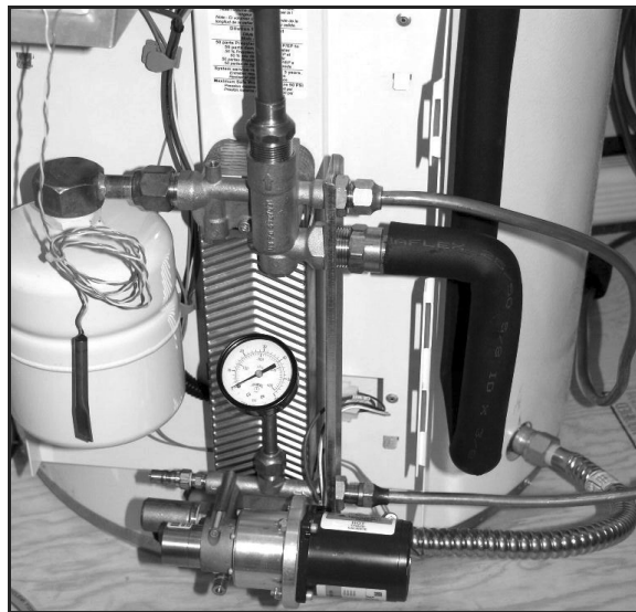
Fig.4.9.1.1 – Line-set connections to Energy Station. Note: For clarity, line-set is not insulated. Proper installation must have insulated line-set to prevent heat loss and to limit burn risk.
