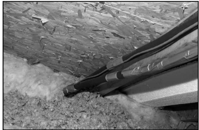
Fig. 4.2.2 – Line-set and control-wire in attic.
