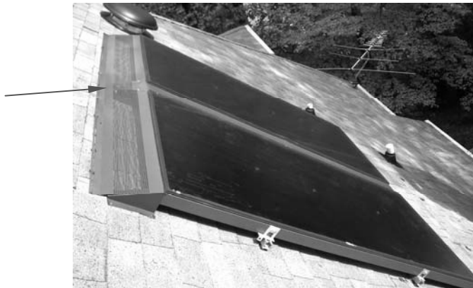
Fig. 7.3.1 – Two collectors with center-flashing and leaf-guard.
