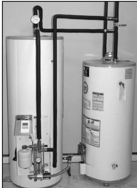
Fig.4.6.1 – All pipes and fittings insulated to limit heat loss and prevent condensation.
