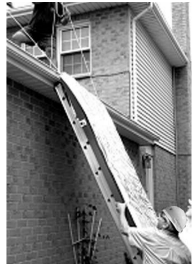
Hoist & Lift Collector
