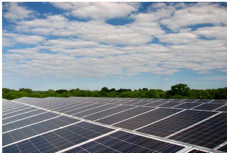
Photovoltaic array at Energy Kinetics' state of the art 64,000 square foot manufacturing facility. Solar power is used to manufacture System 2000.
